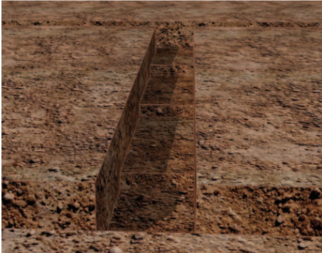
5.13 - Foundation trenches should be dug to a depth of not less than 400mm below the surface all round, following the contours of the ground. The width of the trench is usually twice the thickness of the wall plus 150mm, with a minimum width of 450mm for internal walls. The figure shows how the sides of the trench must be trimmed neatly and square.
