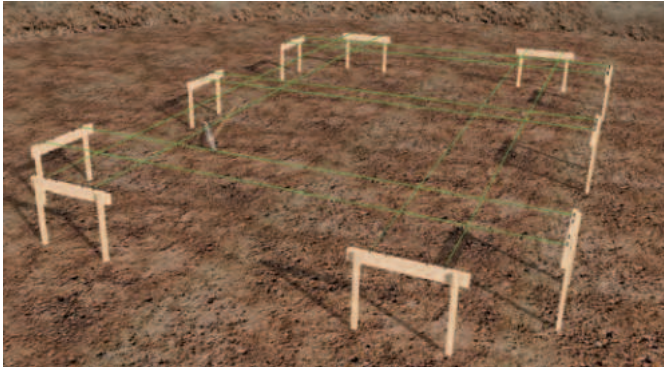
5.9 - The first step in setting out the foundation is to erect timber profile right round the proposed building using scaffolding planks, bluegum poles or any other similar straight timber. All foundations and wall dimensions are then marked out on these profiles by means of nails driven into the wood. The figure shows the builder's line for marking out the foundations.
