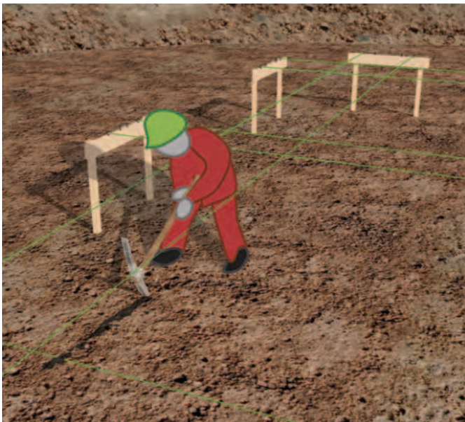
5.11 - The foundation measurements may be transferred to the ground by using a pick as shown
