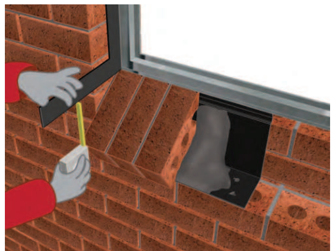
12.18 - Brick-an-edge external sill. The slope of the sill is measured to ensure an equal slope on all the external sills of a particular building. NOTE: The placing of the undersill D. P. C.
