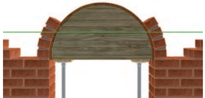
15.5 - Build up evenly on each side to prevent the arch centre from being pushed out of position.
