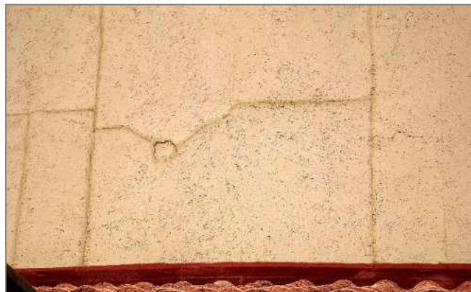
Figure 4 Cracking between pre-fabricated concrete panels and the steel frame due to thermal, moisture and foundation movement.
